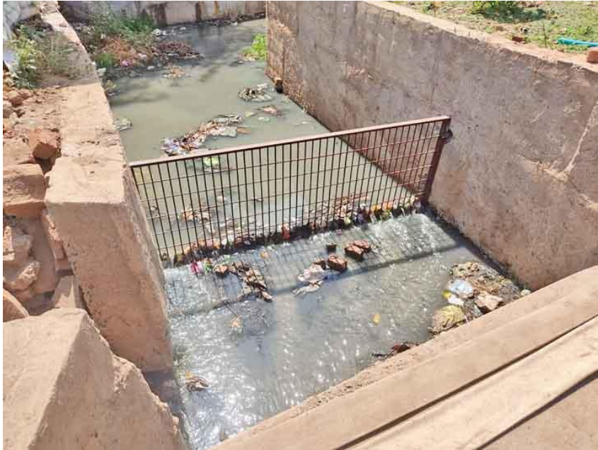
Piliya Nallah Vidisha domestic sewage drains
