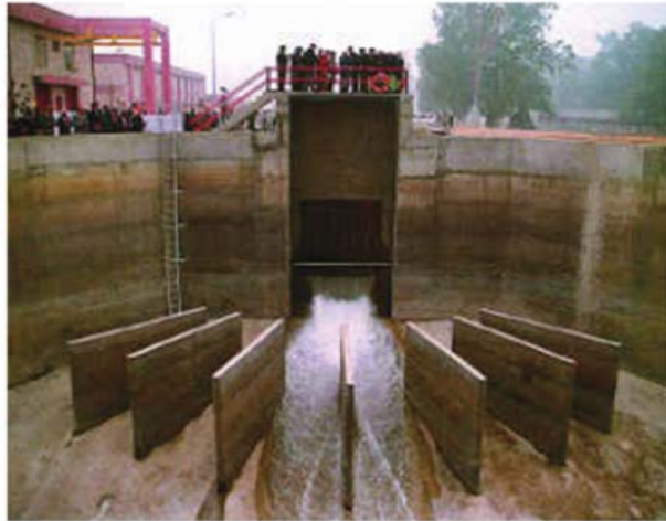
Fig. 18.10 : Water treatment plant
