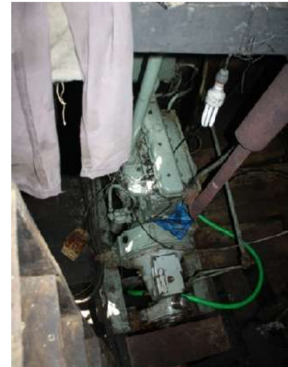
Fig. 11 A view from the upper deck inside the engine room on the lower deck
