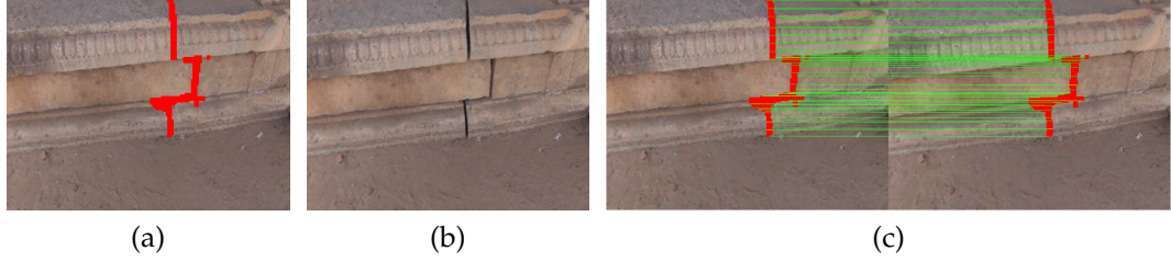
Figure 7.20: Tracking detected regions using the estimated homography matrix. (a) Detected damaged regions in the frame f_{i-1} ; (b) frame f_i ; (c) tracked cracks in the frame f_i . Green lines show the mapping of few points on the boundary of crack regions, while the detected and tracked cracked regions using SIFT features are shown in red.
